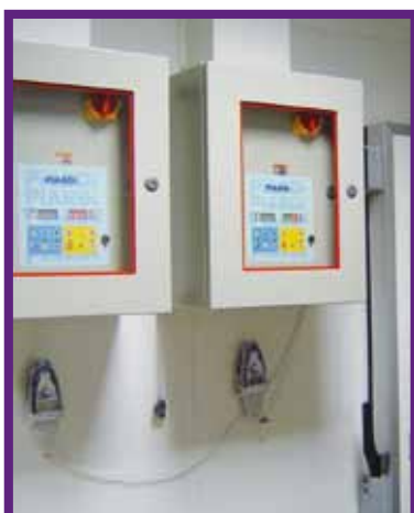
Controllo temperatura in celle frigo
