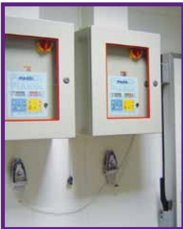
Controllo temperatura in celle frigo
