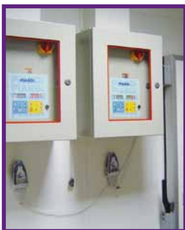
Controllo temperatura in celle frigo
