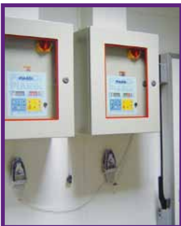
Controllo temperatura in celle frigo
