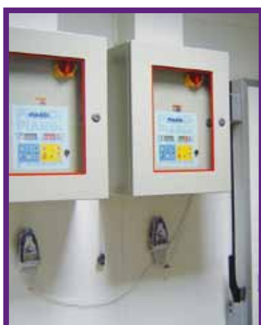
Controllo temperatura in celle frigo
