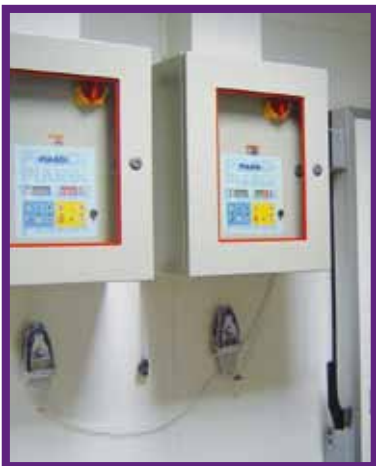
Controllo temperatura in celle frigo
