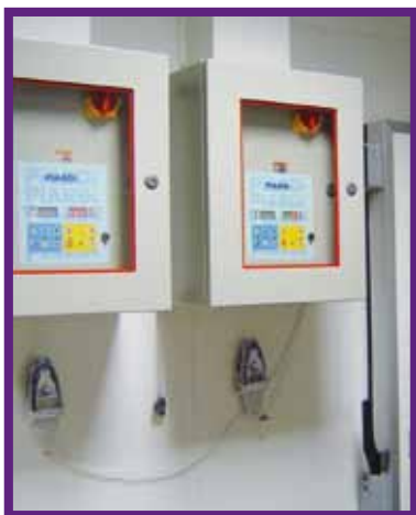
Controllo temperatura in celle frigo
