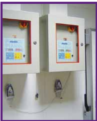
Controllo temperatura in celle frigo
